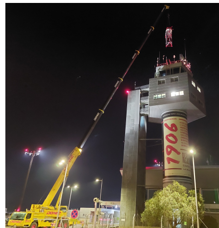
Figura 12: Torre de control remota, Vigo [14]
